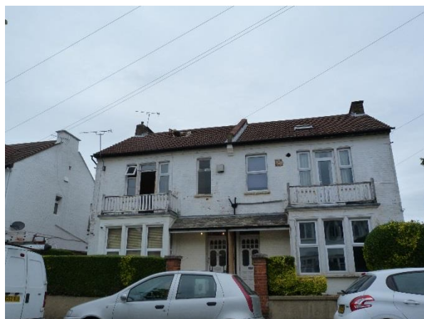
Poor decorative condition of houses on Ditton Court Road, together with inappropriate alterations such as uPVC windows
