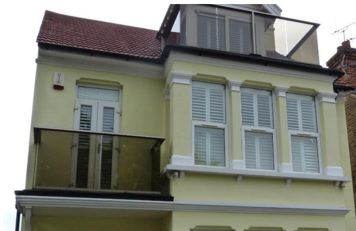
Inappropriate uPVC windows
