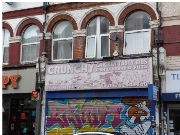
A number of inappropriate features, such as roller shutters, uPVC windows, satellite dishes and plastic downpipes, as well as an example of graffiti
