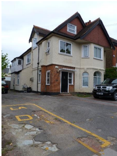
Inappropriate uPVC windows and an unattractive driveway on Preston Road
